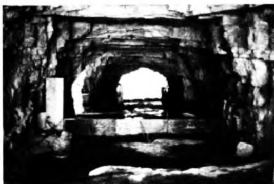
Fig. 4. Photo showing the disposition of the sandstones at the downstream portal of Tunnel I
